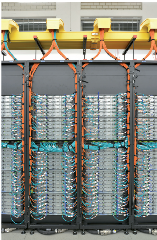
Figure 5: Several racks of SuperMUC Phase 2.
