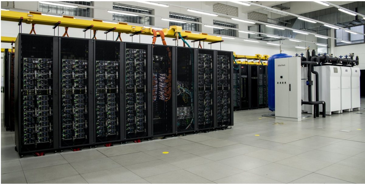
Figure 2: CoolMUC-2 (left) and adsorption chiller (right). Picture: Michael Klinskyk.
