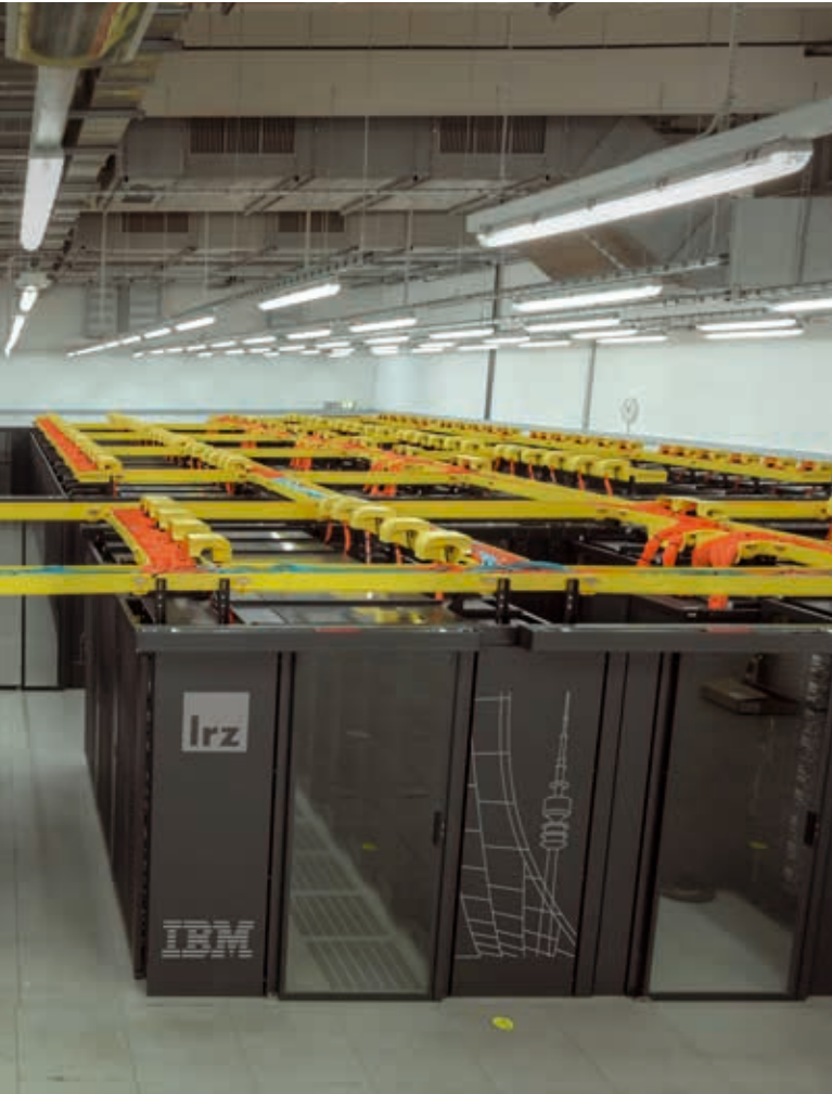
Picture of SuperMUC in the server room. The yellow cable trays on top of the racks contain the cables for the Infiniband interconnect.
