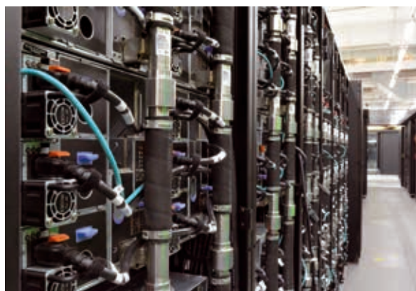
Figure 4: Rear of racks with warm water cooling.
