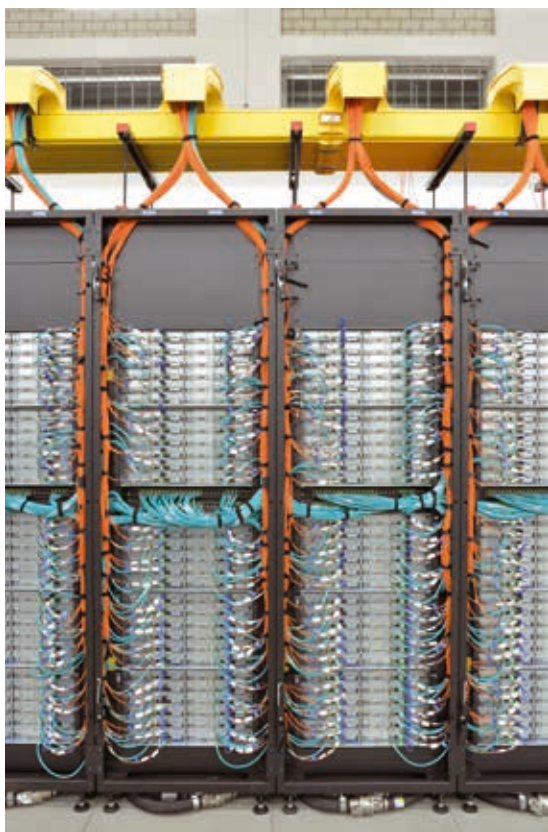
Figure 5: Several racks of SuperMUC Phase 2.
