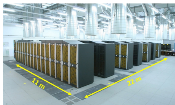
Figure 2: SGI Altix in the new computer room of LRZ.
