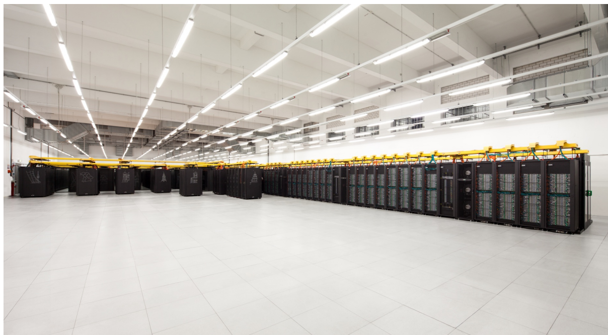
Figure 1: SuperMUC Phase 1 on the left and SuperMUC Phase 2 on the right, in the server room.
