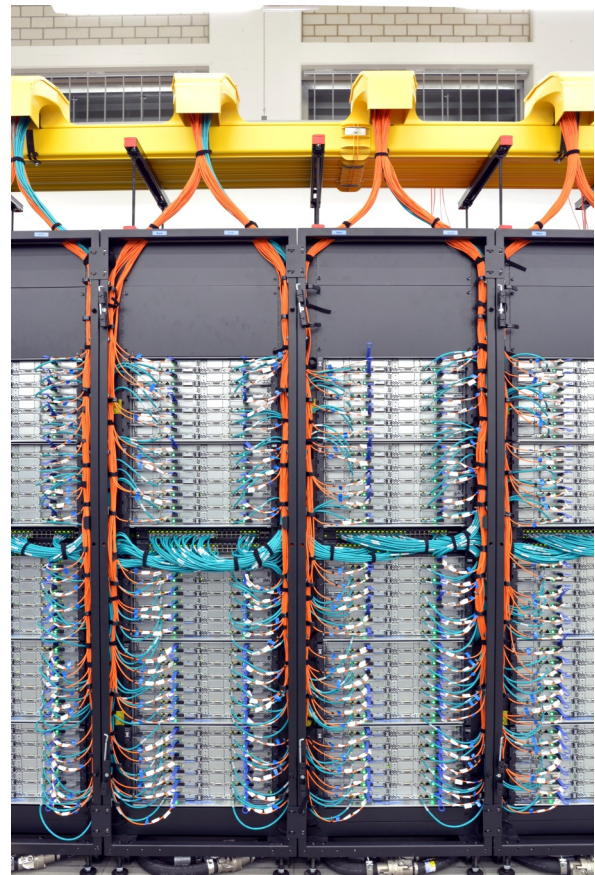
Figure 6: Several racks of SuperMUC Phase 2.
