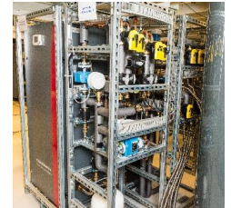
Booster Heat Pump Transfer Station
