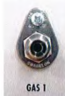
gas connection on machine
