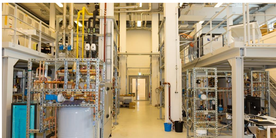
Figure 3: Front view of the CoSES lab with an experimental bidirectional heat network
