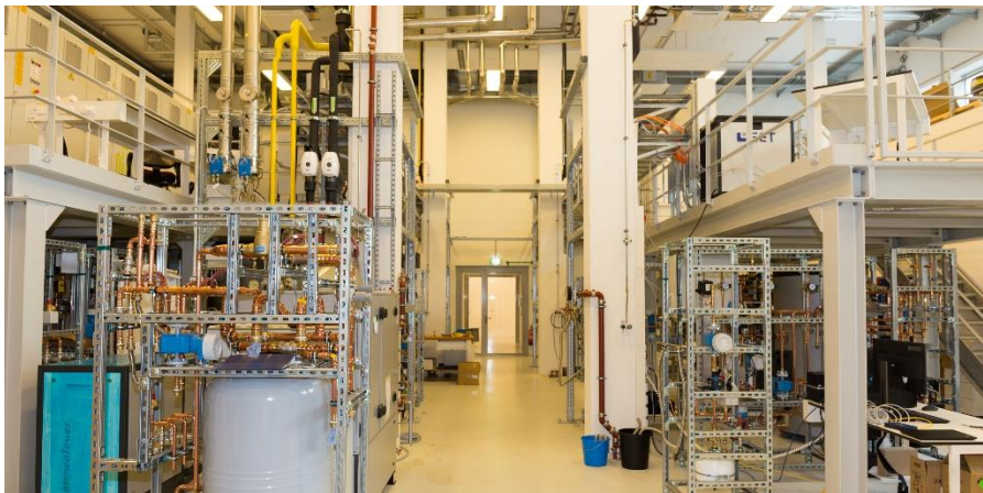
Figure 1: Front view of the CoSES lab with an experimental bidirectional heat network
